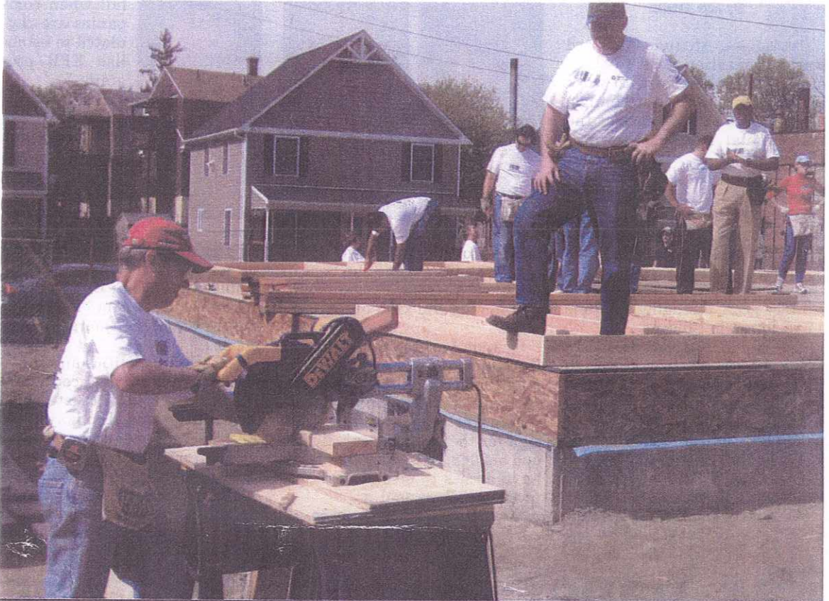
MEASURE TWICE, CUT ONCE: Volunteers help construct two homes being built by Habitat for Humanity in Hartford, Conn. Oakleaf Waste Management is donating roll-off containers and employing a single-stream recycling system for the project.
